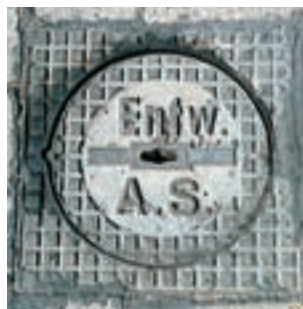
Fitting Found on roads or footpaths, used for shutting off or opening wastewater pressure pipes. The green sign indicates their position.
