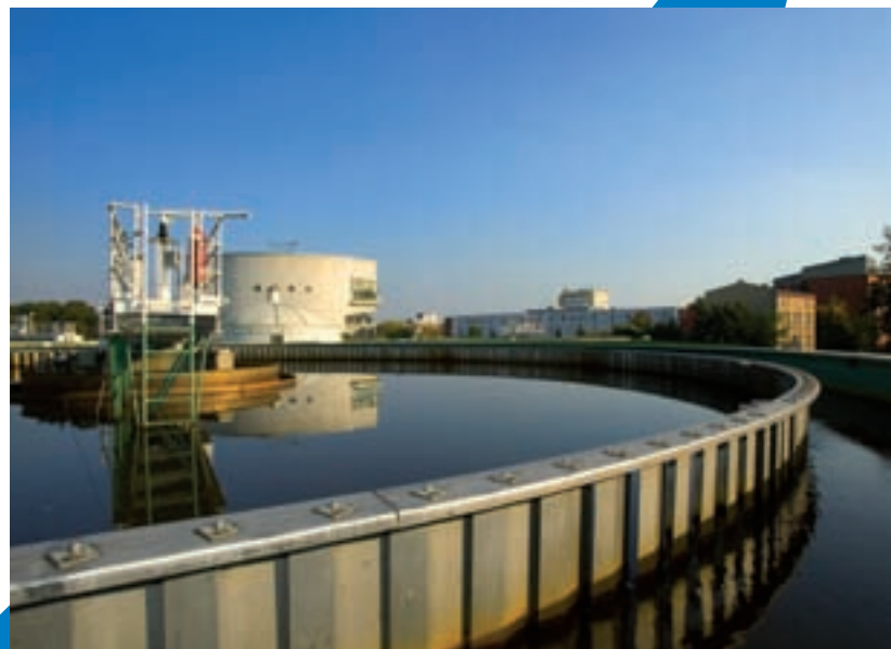
Surface water treatment plant in Tegel
