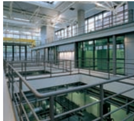
Wastewater pumping station Hohenzollerndamm
