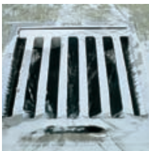
Road gully Rainwater and other water from the road is carried into the stormwater or combined sewers through the road gullies. Any solids carried along in the water settle in the silt chambers.
