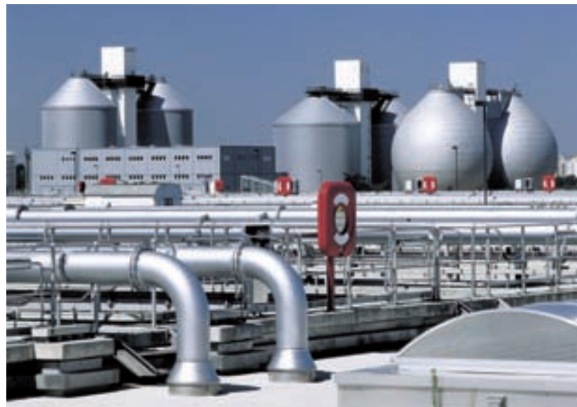
Aeration tanks, in the background digestion tanks
